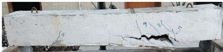
Fig. 9. SB2 Beam failure.
