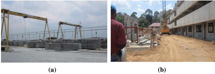
Fig. 4. (a) Production yard for the integrated wall/column panels, (b) Construction site of the hostel.
