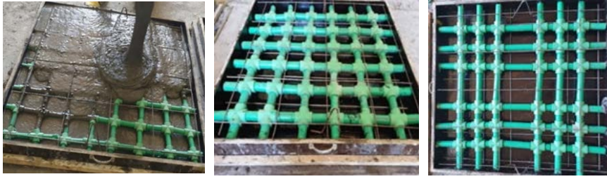
Fig. 1. Constructing two-way hollow reinforced concrete slabs using two-way piping systems of plastic pipes and fittings.
