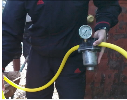
Fig. 2. Biogas Sampling Line.
