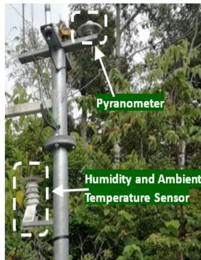
Fig. 4. The used weather station installed in the solar research site to measure the weather parameters.
