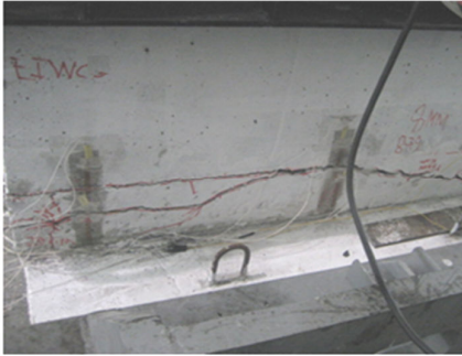
Fig. 13. EIWC3 Specimen at Failure.
