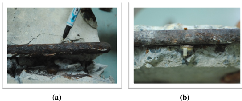
Fig. 12. Visual Inspection of Corroded Rebar: (a) Specimen Exposed to Indoor Environment. (b) Specimen Exposed to Corrosion Chamber.
