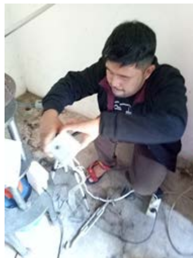
Fig. 5. Implementation of the radon monitoring system.
